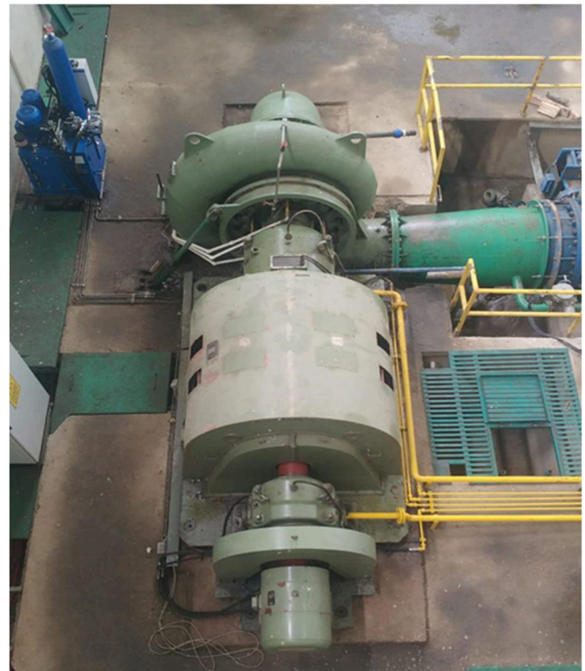
Fig. 3. A generation unit installed on a hydroelectric power plant
