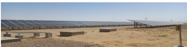
Fig. 1. Photovoltaic plant of Tozeur 2.
